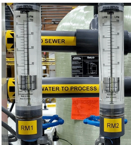
Visual flow meter.
